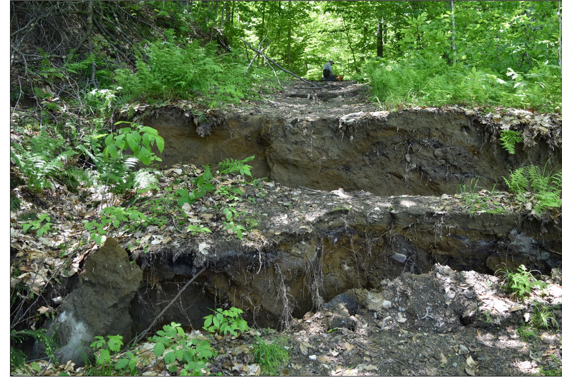
Fig. 2. June 12, 2019: Ground cracks and scarps due to rotational failure along landslide margins. Foster's Trail ended abruptly.
